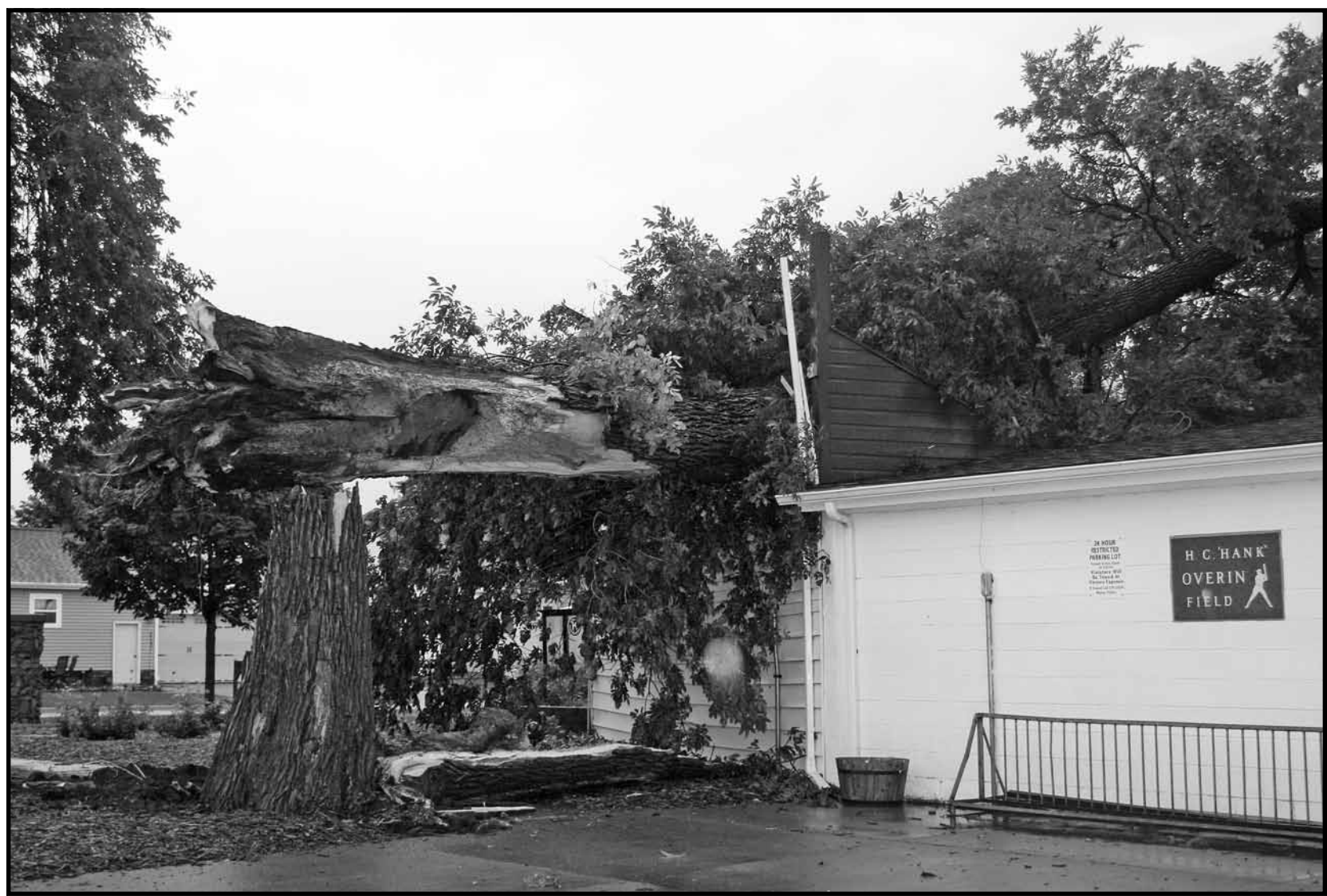
As high winds in excess of 90 miles per hour rolled through Wayne, an old ash tree sitting near the front entrance of Hank Overin Field was split and lifted out of the ground before being dropped on the grandstand at the facility, which was built during the Great Depression in the 1930's.
